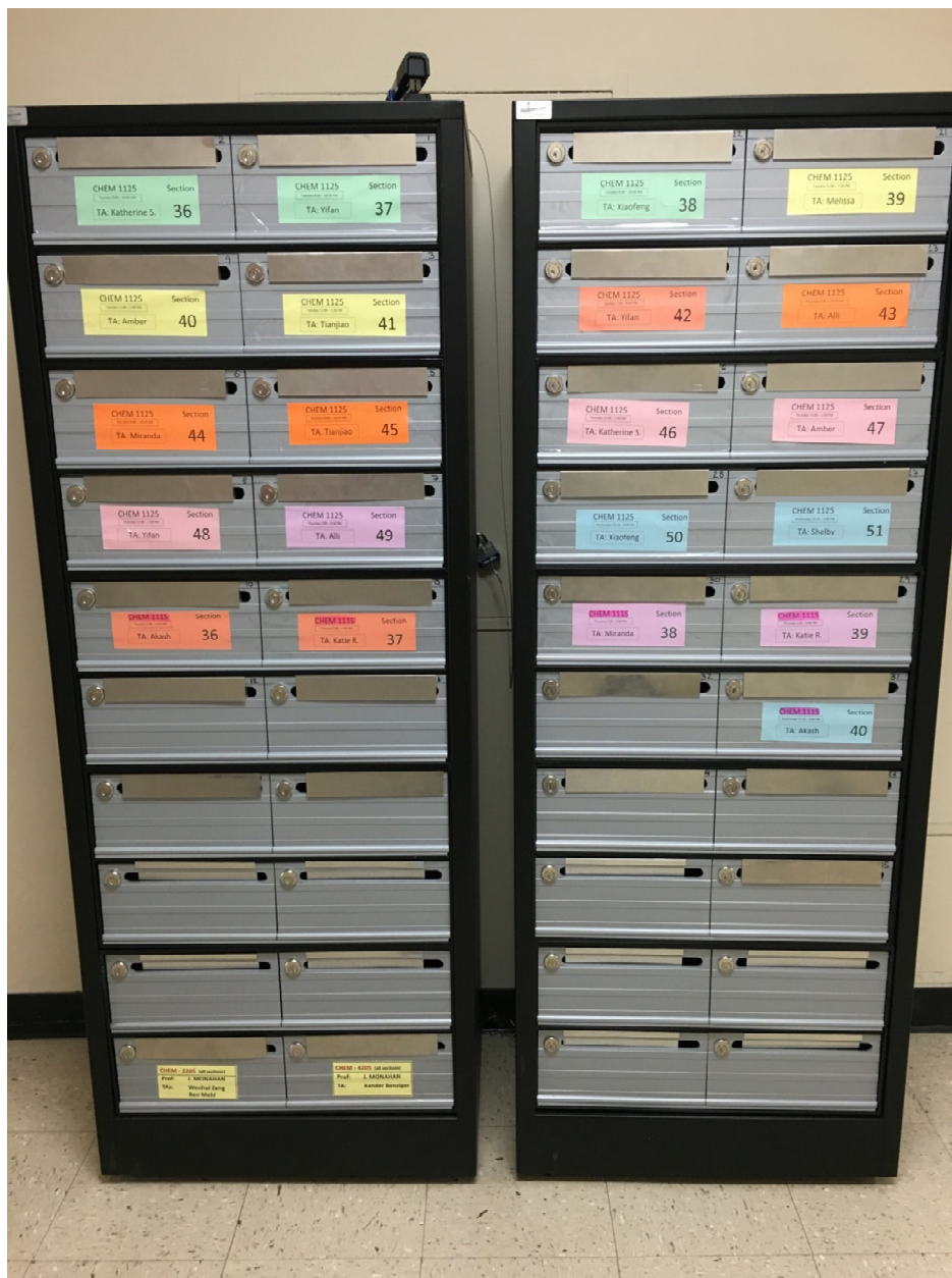
Figure 1a: Installed Mailbox System, Monsanto Hall
